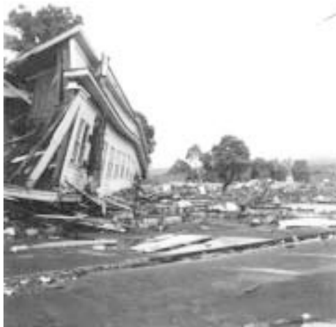
Damage to building in Hilo, Hawaii, from the 1960 tsunami. Although there are engineering techniques and materials that can be used to resist tsunami forces and inundation, in cases of intense tsunamis, they will reduce losses but not prevent severe damage. Credit: Pacific Tsunami Museum
