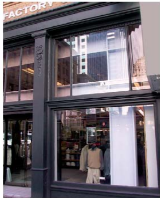
Steel moment frame for a commercial retrofit. The large (white) double frame is placed behind the original façade columns.
