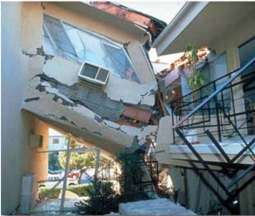
California earthquake damage.
