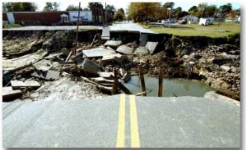
Damage to a highway.
