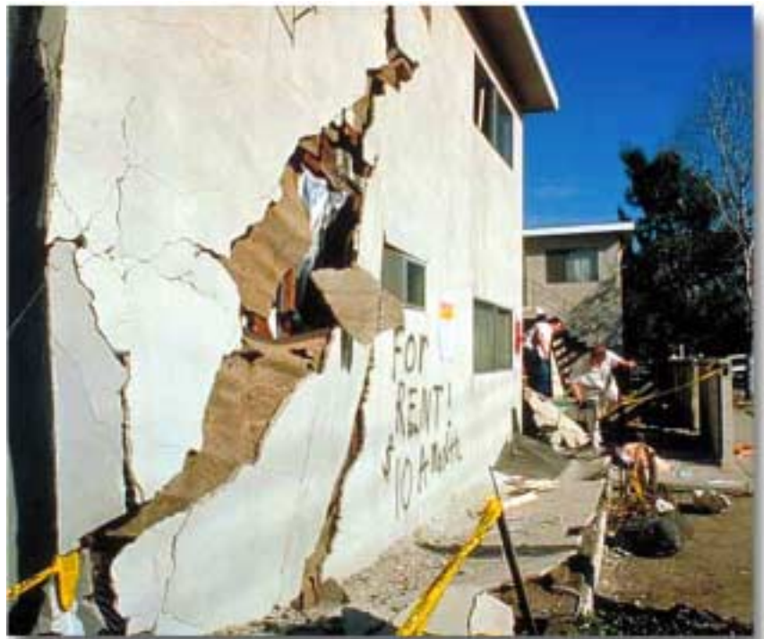
California earthquake damage.
