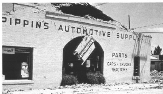
Small businesses in older unreinforced brick or masonry buildings are among the hardest hit in an earthquake.
