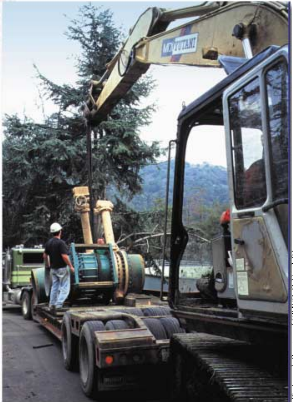
EBMUD installed remote-control shutoff valves at water treatment plants to preserve the water stored there for post-earthquake uses, such as fire fighting.
