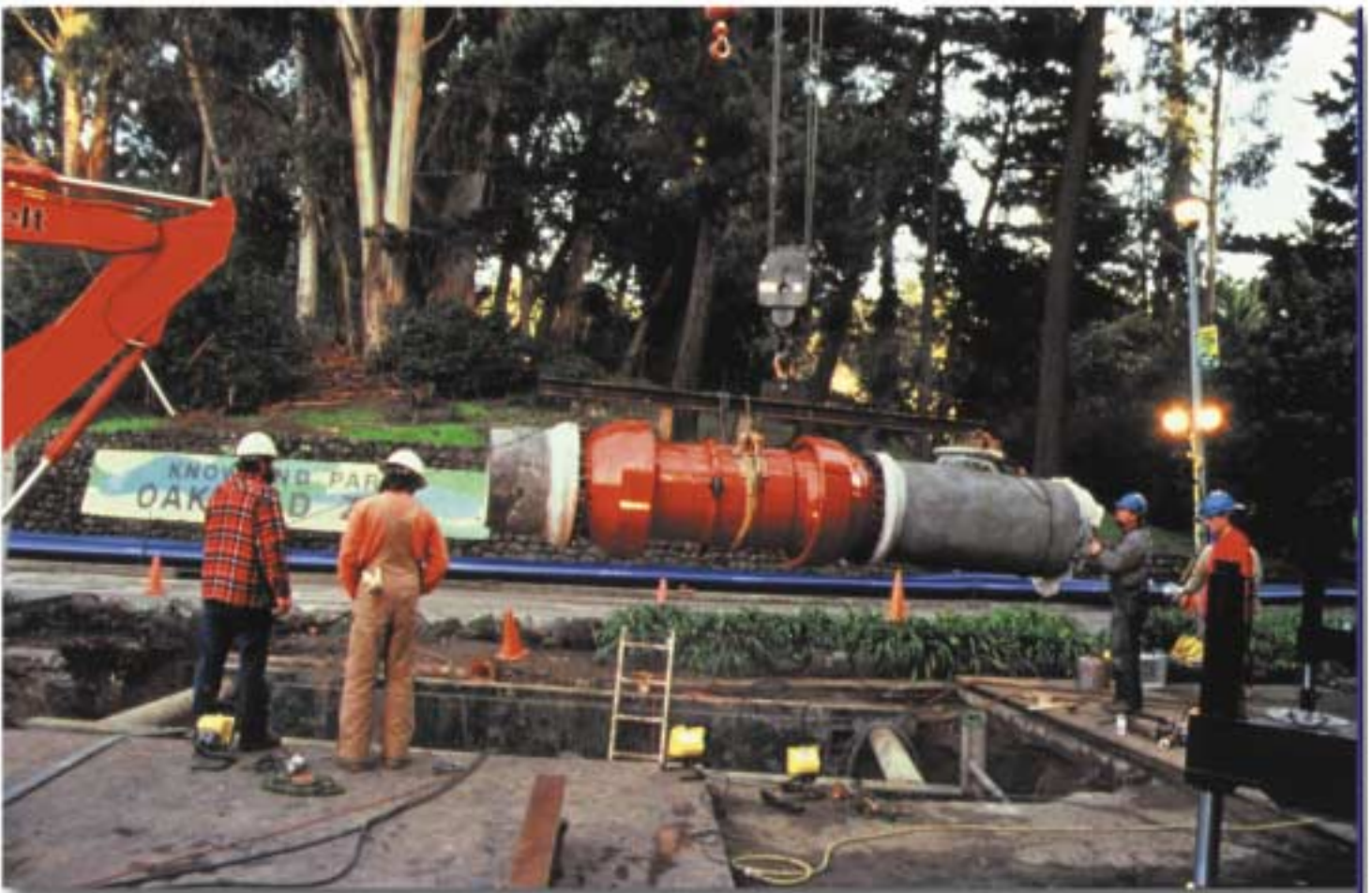
An EBMUD contractor installed a flexible pipe joint in an area experiencing "fault creep" near the entrance to the Oakland Zoo.
