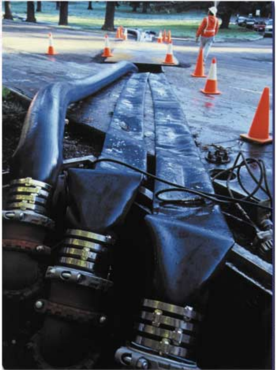
Flexible hoses can bypass sections of broken water pipes. This innovative solution to seismic risk will allow quick restoration of service and vital fire fighting capacity.
