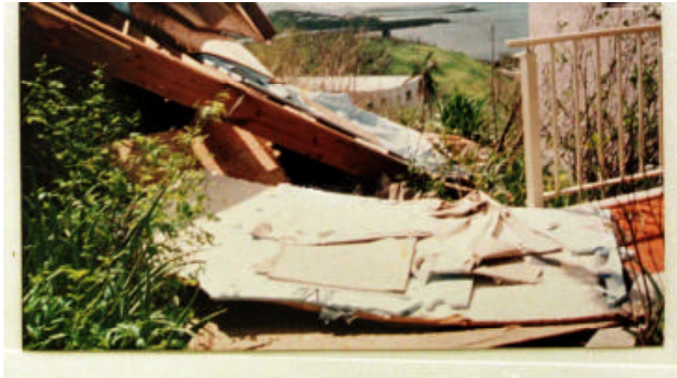
High winds generated by Hurricane Georges caused a partial collapse of this building.
